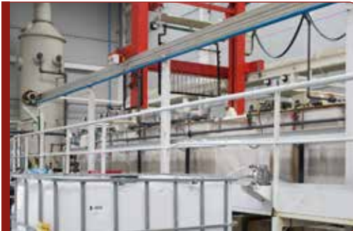
PROCESS WATER / SURFACE TREATMENTS / WASTEWATER
